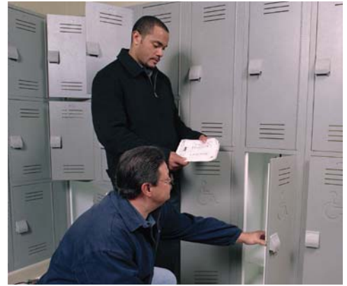
The Chicago Park District's Anthony Hayes and Larry Cirincione of Division 10 Supplies take a closer look at the new locker installation at Independence Park.
