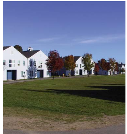
Bradley TMVs installed in the University's seven student apartment clusters help control water temperatures and provide scald protection for students.
