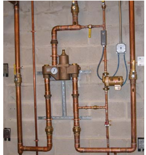
Navigator TMVs are designed to fit virtually an application, and can be easily retrofitted for an existing system like the one at NovaCare Complex.
