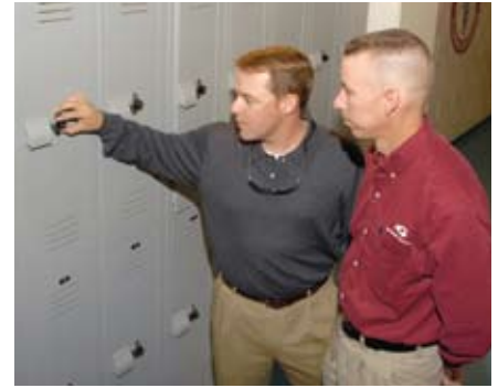
Mike McLeod (left) and Mike Hurst take a closer look at a few installed lockers.
