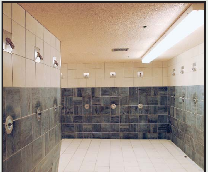
By changing to Bradley showers with Touch Time controls, West Edmonton Mall has saved on maintenance repairs and energy costs.
