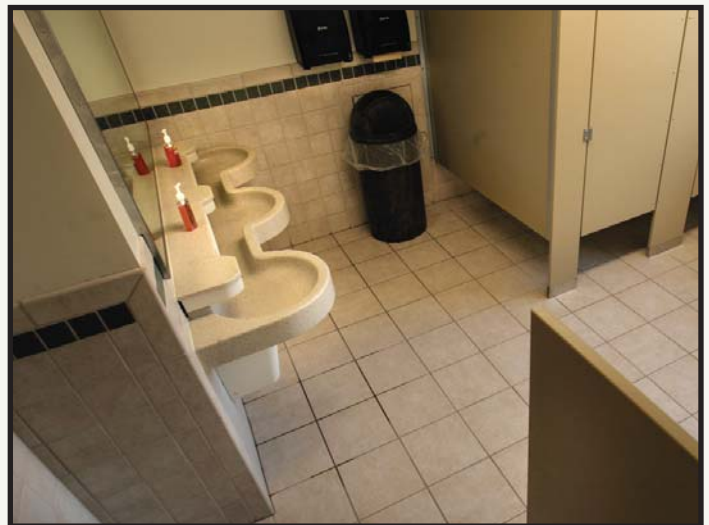
The three-station SS-Series Express® Lavatory System in the boy’s restroom is extremely durable and has significantly reduced maintenance time and costs.
