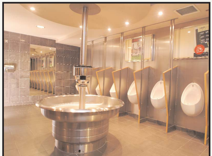
A Bradley Circular Classic Washfountain in stainless steel serves as the visual centerpiece of the men's washroom at Lloyd's No. 1, The Trafalgar. The washfountain is as economical as it is practical for the washroom's design - the unit accommodates up to eight users at one time.
