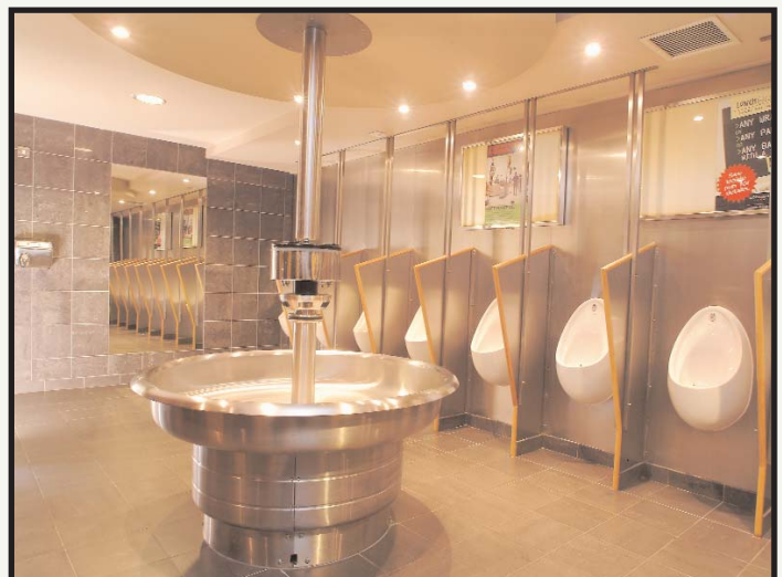
A Bradley Circular Classic Washfountain in stainless steel serves as the visual centerpiece of the men's washroom at Lloyd's No. 1, The Trafalgar. The washfountain is as economical as it is practical for the washroom's design - the unit accommodates up to eight users at one time.
