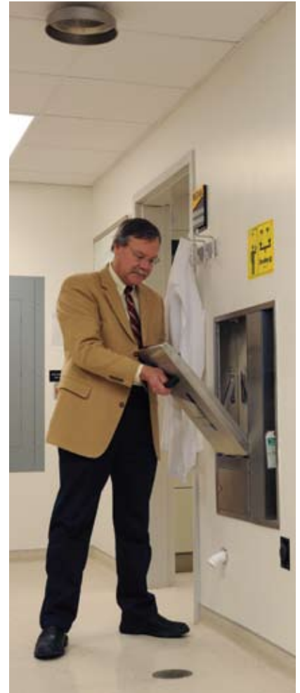
Jon Krezoski inspects one of the science lab's recess-mounted emergency fixtures. Jon and his facility team at Lapham Hall appreciate that the new drench shower/eyewash units are easier to test and maintain. The old units were "vintage 1960s" with no floor drains for the shower.
