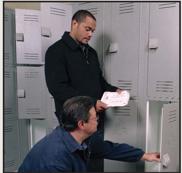
The Chicago Park District's Anthony Hayes and Larry Cirincione of Division 10 Supplies take a closer look at the new locker installation at Independence Park.
